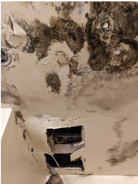
Mold on barracks ceiling.
